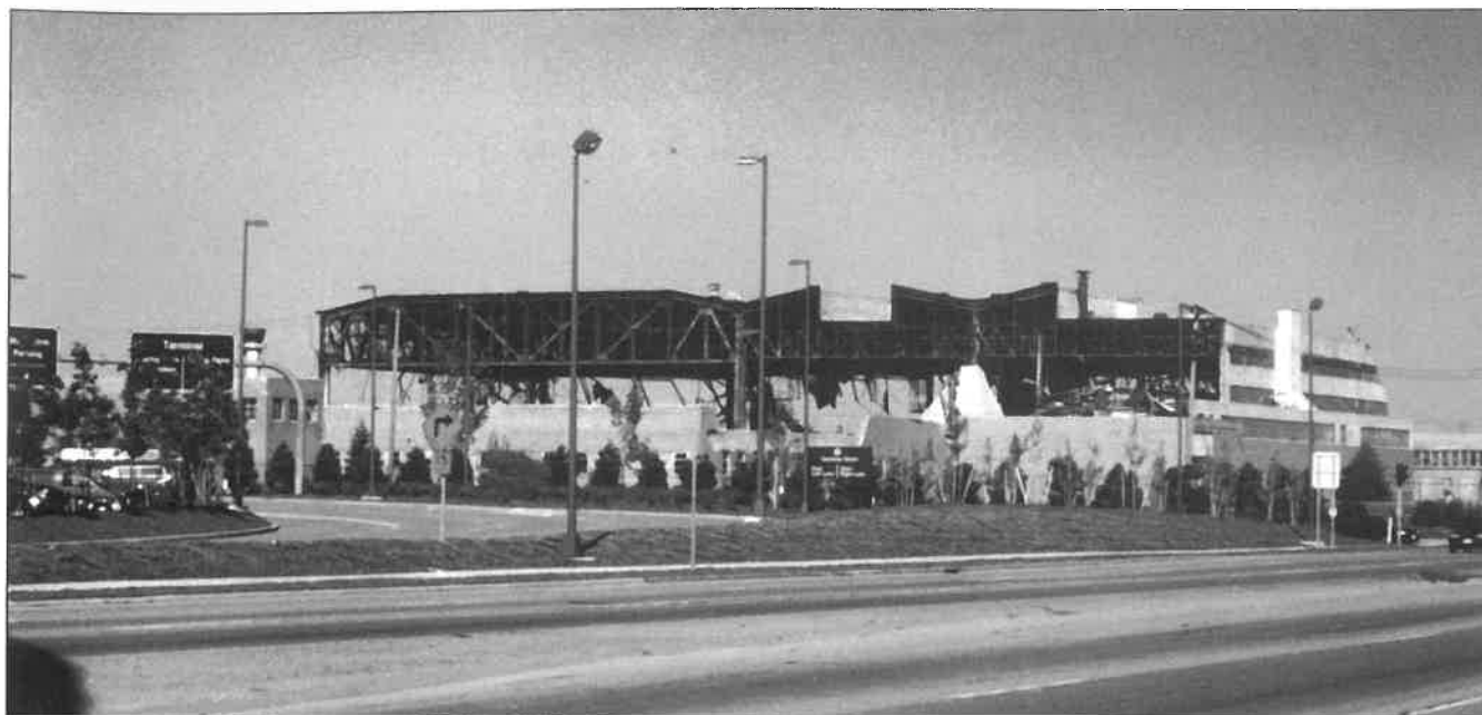
Westinghouse Plant demolition (from the southwest) showing the structural steel framing of the Albert Kahn building with the moderne style administration building at the right.
